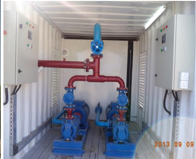
WATER PUMP UNIT
